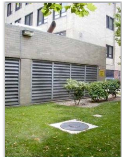
Figure 4-1. Air Intake Vent
