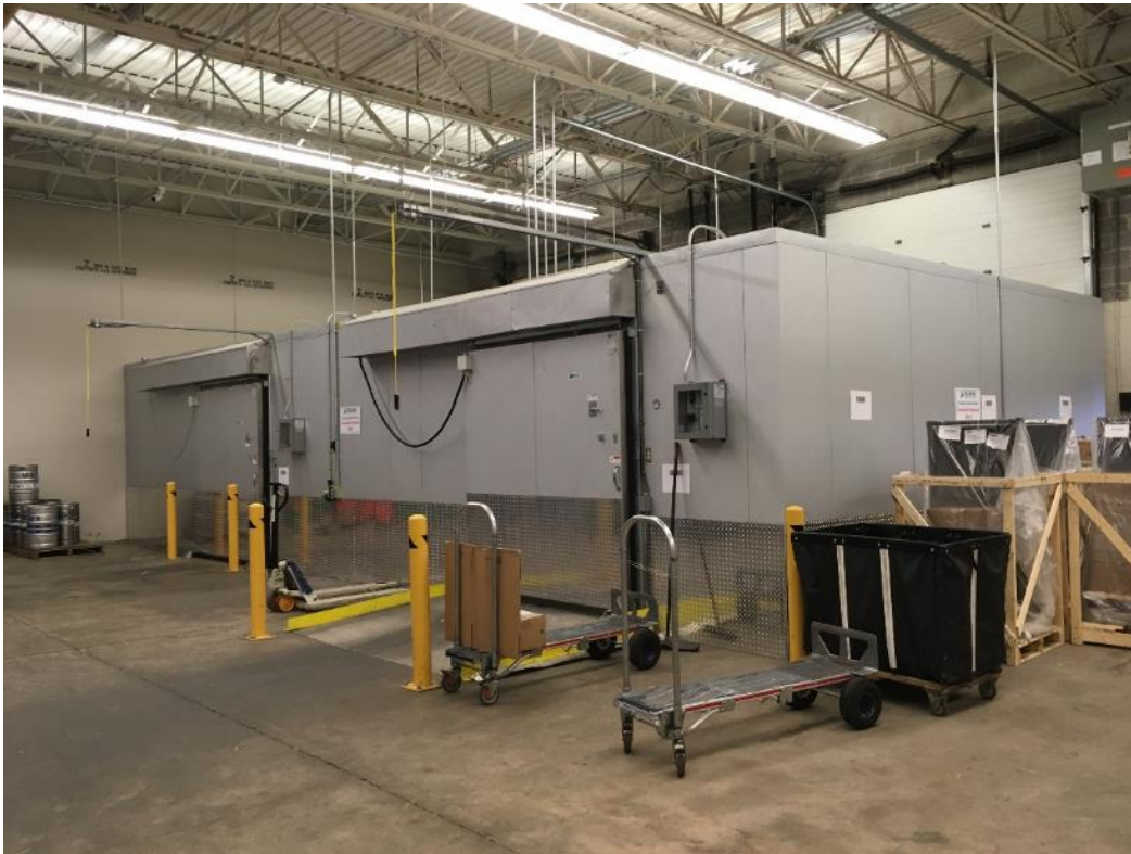
Figure B-18. Case Study 2: Cooler and Freezer in Warehouse
