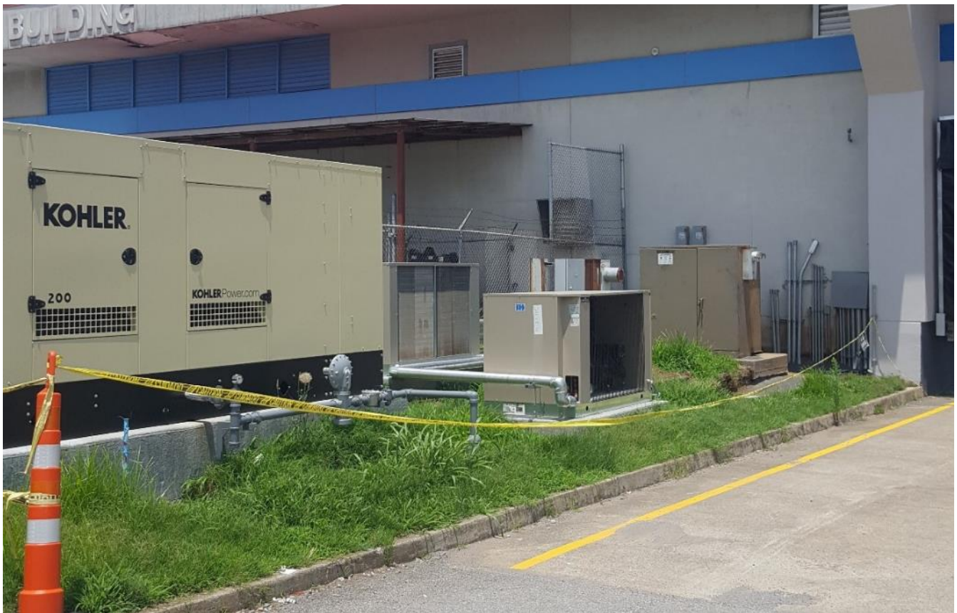
Figure B-45. Case Study 4: Emergency Power Generator
