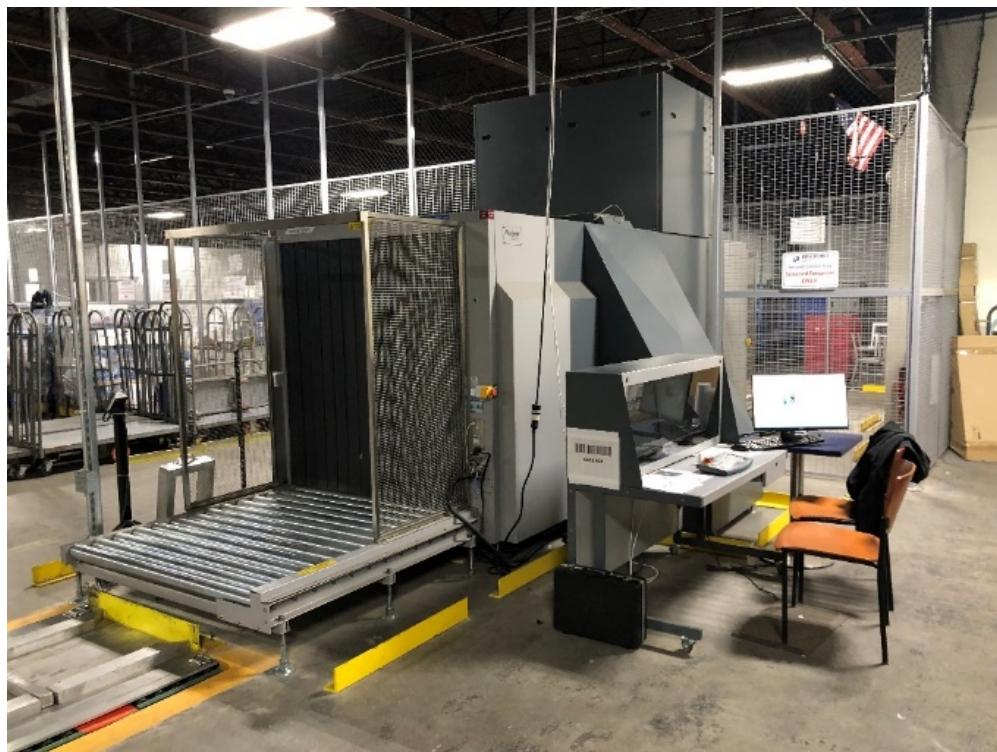
Figure B-5. Case Study 1: Screening Equipment
