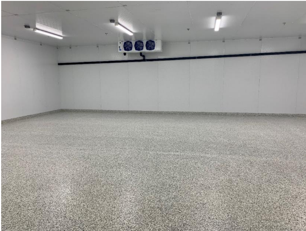
Figure B-29. Case Study 3: Cooler and Freezer in Warehouse
