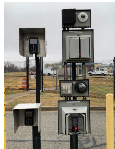
Figure 6-1. Bi-Level Access Control Panel
