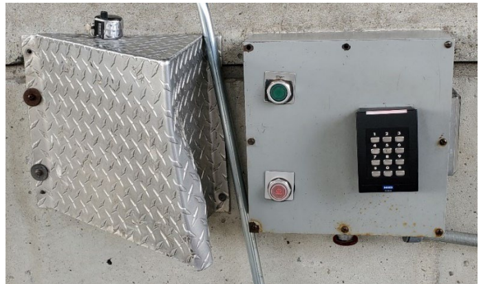
Figure D-15. Damaged Wedge, Undamaged Control Panel
