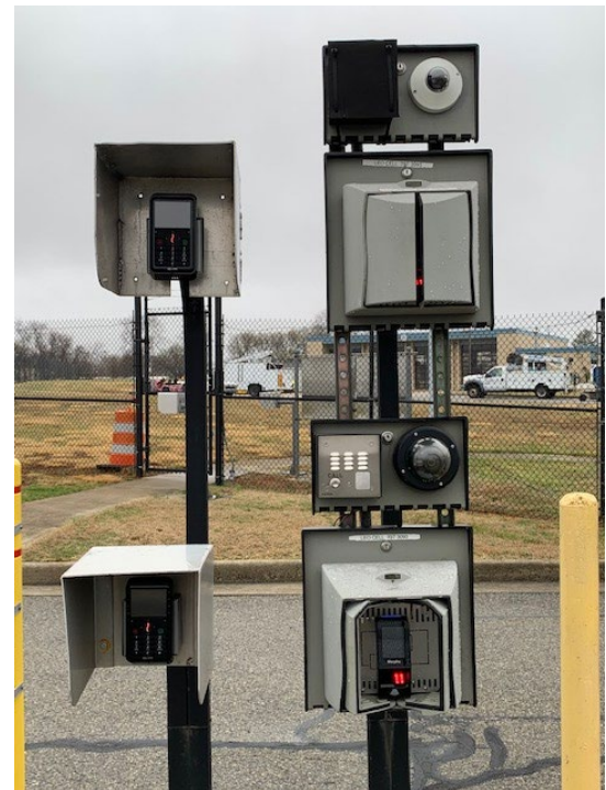
Figure C-3. Two-Tiered Access Control Panel with Camera and Fingerprint Reader
