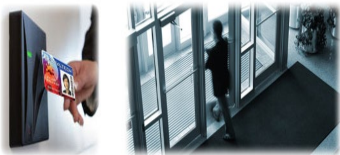
Figure 5. Badge and Card Reader Access Point
