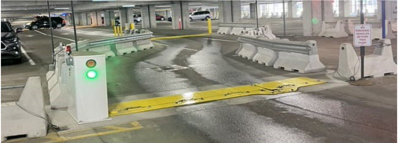
Figure A-23. Steel Guardrails Affixed to Concrete Barriers
