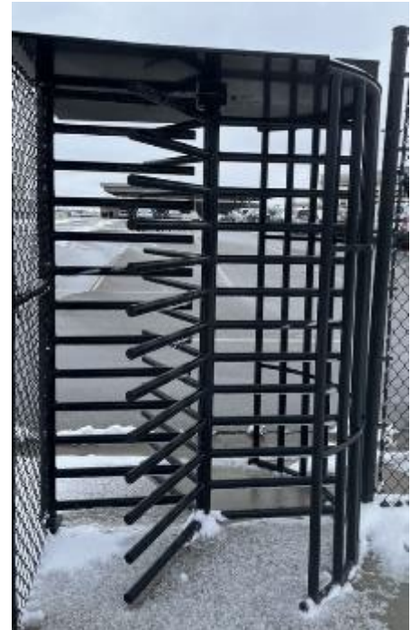
Figure 8-16. Full-Height Pedestrian Turnstile Access Door
