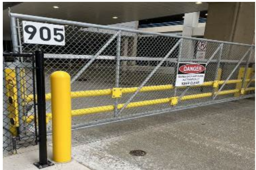
Figure A-24. Fire Lane Slide Gate
