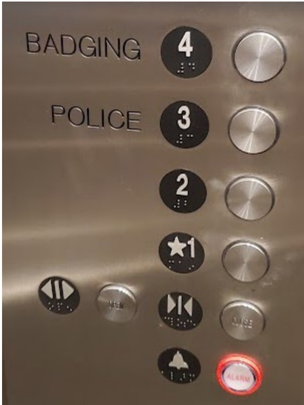
Figure 4-52. Elevator with Office Label
