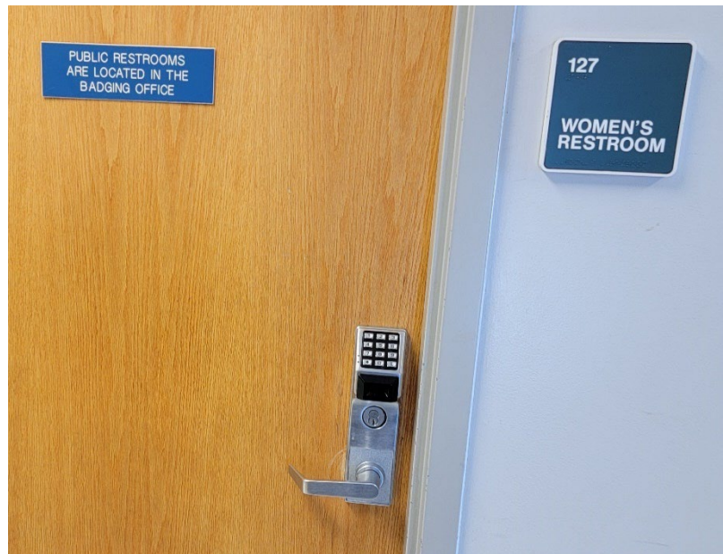
Figure 4-30. Restroom with Access Control
